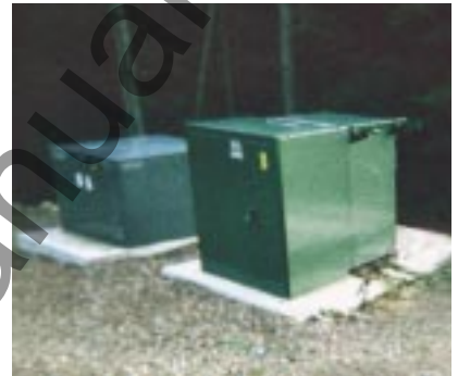
A "traditional" transformer/switchgear combination.
