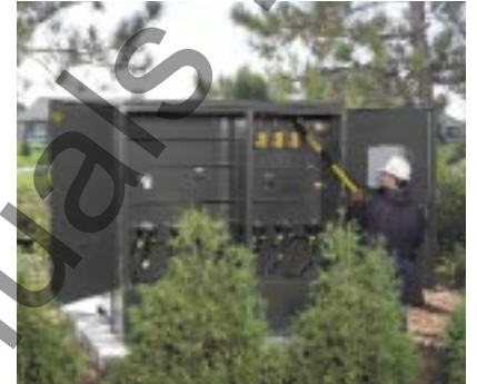
Combining VFI switchgear and a transformer in a single enclosure is more aesthetically pleasing in a residential setting.
